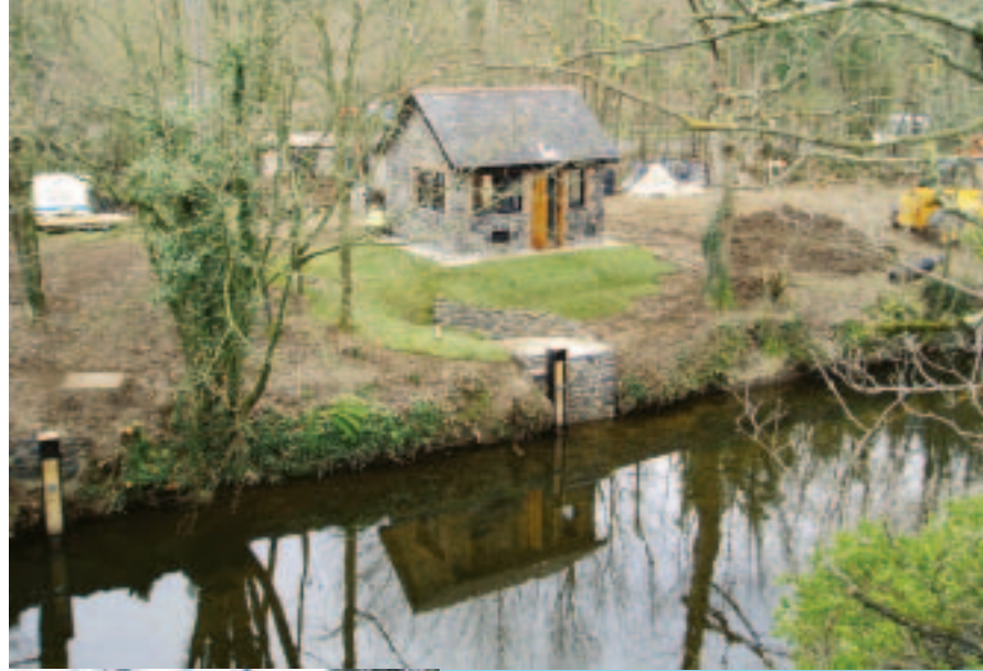
River flow measurement application showing the transducers in crossed path configuration, mounted on vertical piles.
